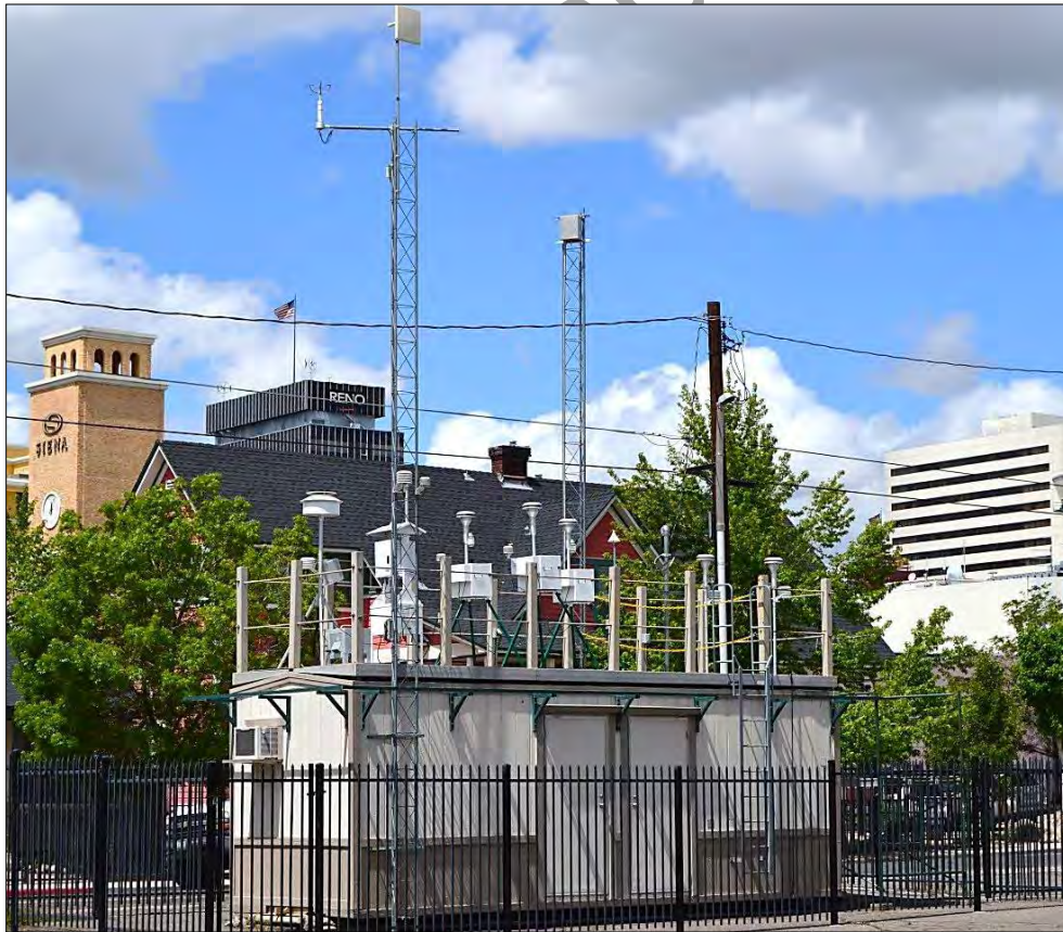
Figure 10 Reno 3 Monitoring Station
