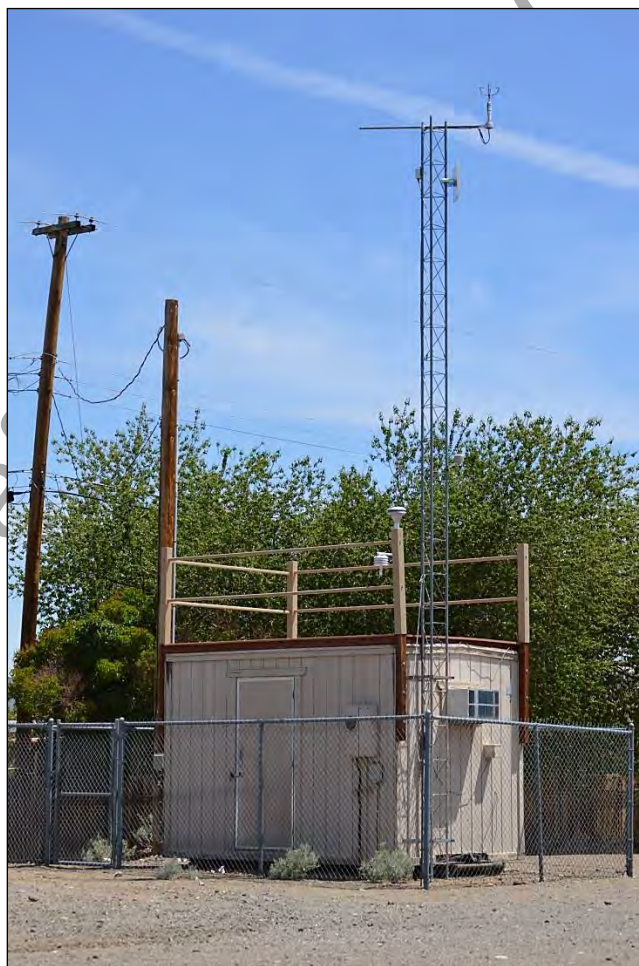
Figure 8 Plumb-Kit Monitoring Station
